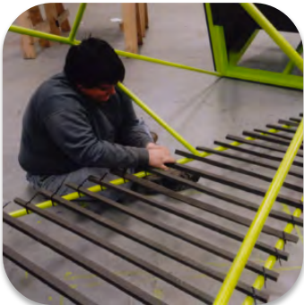
Placing the siding on ChickTopia coop's chicken run, 2011. Photo: Project H Design.
